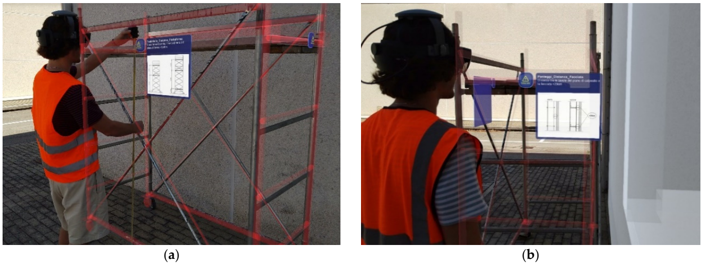
Figure 9. Checking the height of the scaffolding's first-level deck above the ground (a) and the distance from the wall prescription (b).
