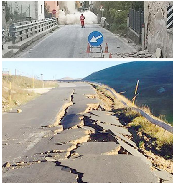
Fig.4 Marche Region, Visso (MC), Damage to infrastructure caused by the 2016 Central Italy earthquake. Source: Visso municipality, Marche Region
