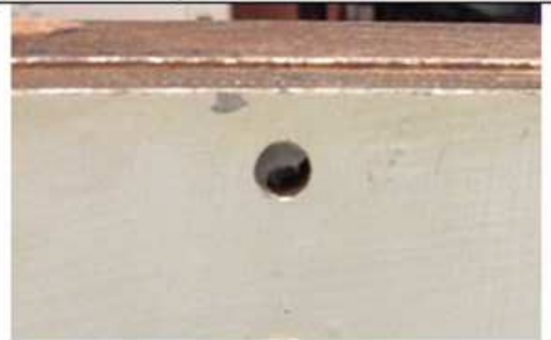
c) Circumferential defect
