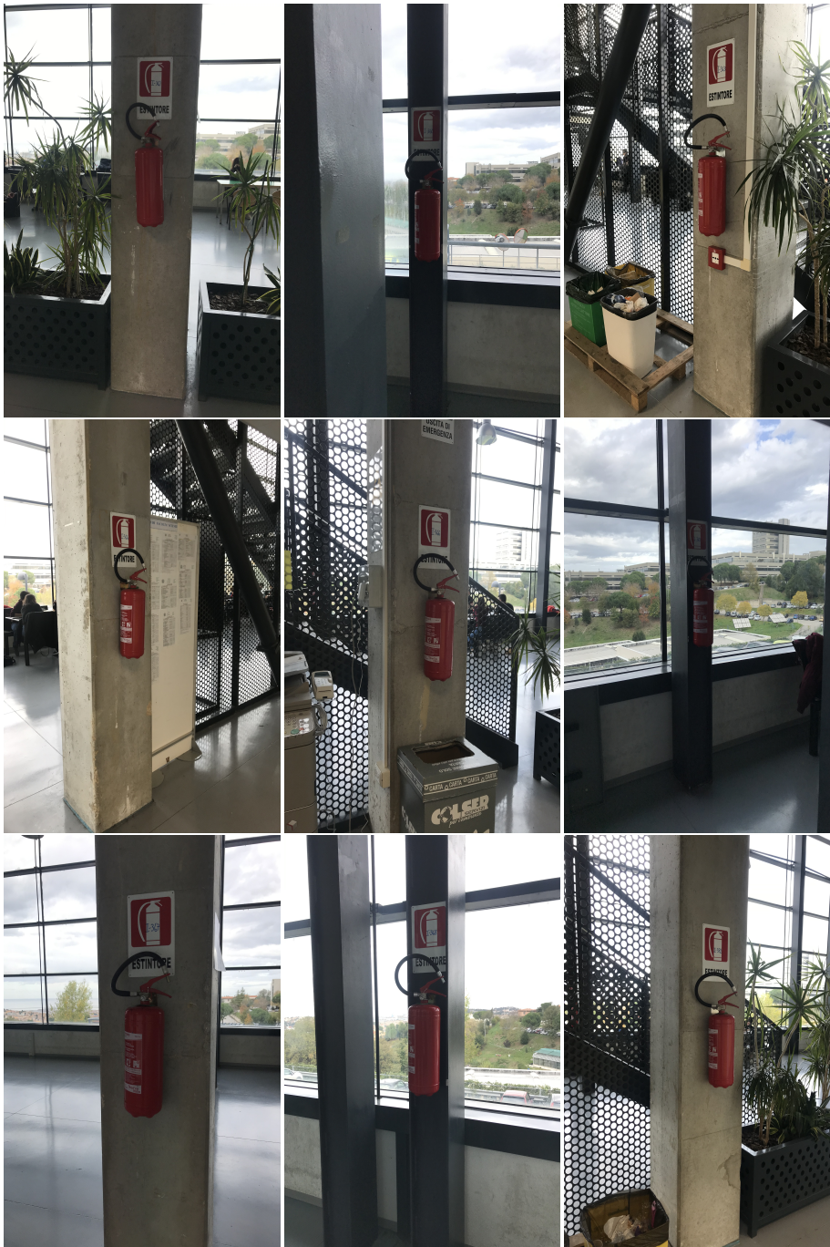
Figure 5.17: Fire extinguishers point of view during BAS test, ground floor. First row, left to right FE1, FE2, FE3. Second row FE4, FE5, FE6. Third row FE7.
