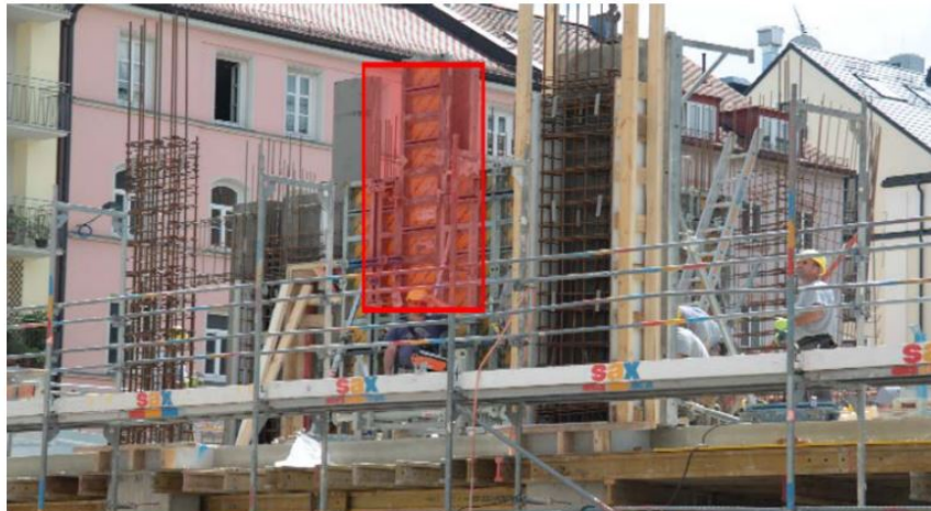
Figure 2.17: Detected bounding box for formwork elements on a photography of a construction site [Braun et al., 2019].
