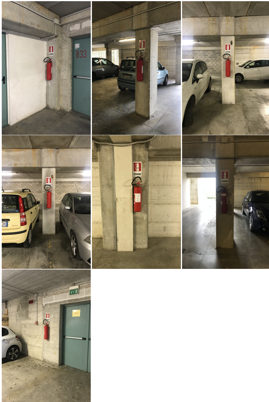
Figure 5.16: Fire extinguishers point of view during BAS test, basement floor. First row, left to right FE1, FE2, FE3. Second row FE4, FE5, FE6. Third row FE7.
