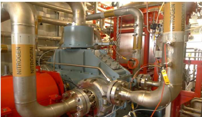
(b) Internal view of power container of the LAES pilot-plant
