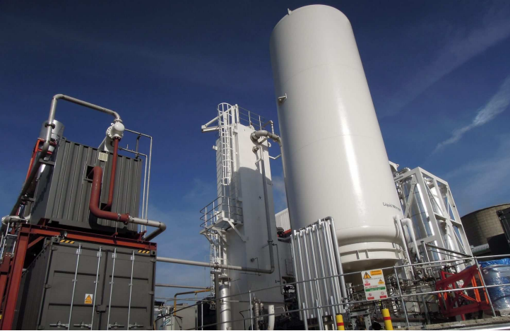
(a) External view of the LAES pilot-plant
