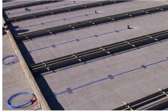
Figure 2.6. Installation of embedded electrodes and monitoring system in a self-heating concrete pavement [67]
