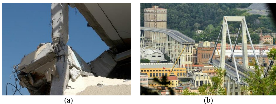
Figure 7.1. a) Seismic damage of a reinforced concrete structure (crisis of the pillar-beam node), b) Morandi bridge (Genoa, Italy) after collapse (August, 2018)
