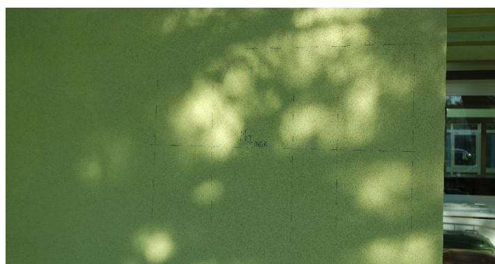
Figure 4.10 A pacometric test on a RC wall to verify the positioning of steel bars (Brugnetto – Ripe).
