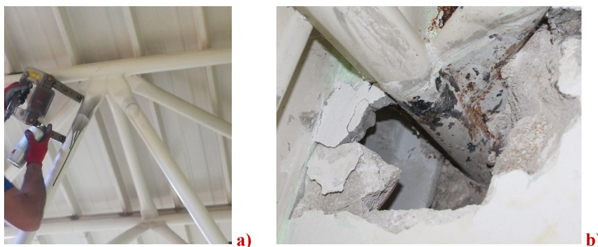
Figure 4.13 A magnetoscopic survey for the detection of defects (a) and the evaluation of the degradation on metallic elements (b) (Ponte Rio - Monterado).
