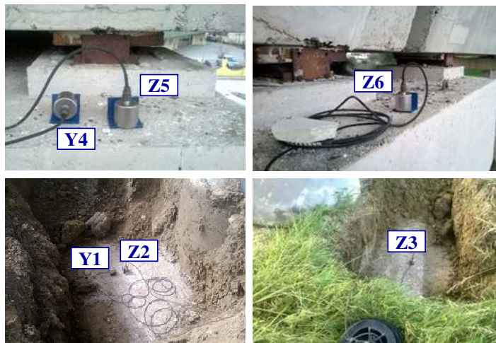
Figure 4.16 Accelerometers photos placed in P3 Configuration
