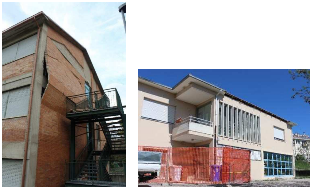
Figure 8.17. Damage to masonry infills (left) and to roof eaves (right)
