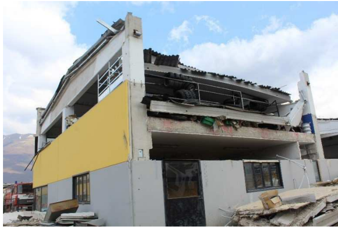
Figure 1.6. Partial collapse of a pre-cast RC industrial building (Norcia, 2016 Centre Italy earthquake)
