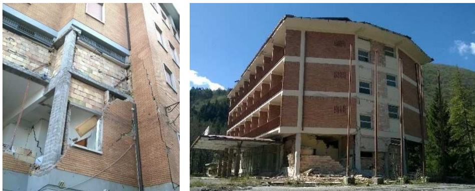
Figure 8.9. Damage to masonry infills in the municipalities of Urbino (left) and Norcia (right)
