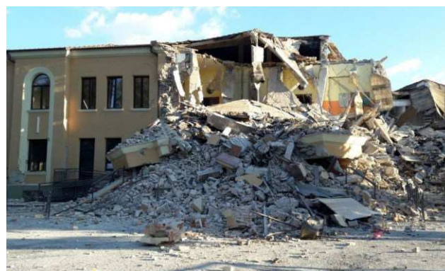
Figure 4.1. Collapses of school buildings: San Giuliano di Puglia, 2002 (left) and Amatrice, 2016 (right).
