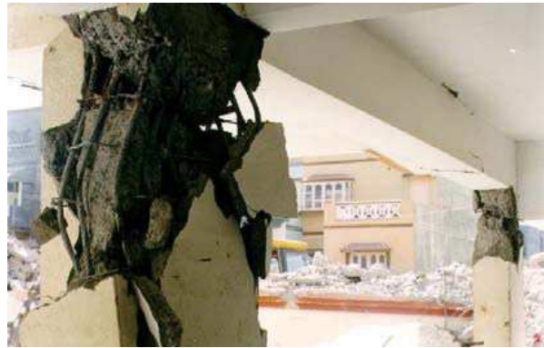
Figure 1.13. Shear failure and concrete crushing failure in concrete columns
