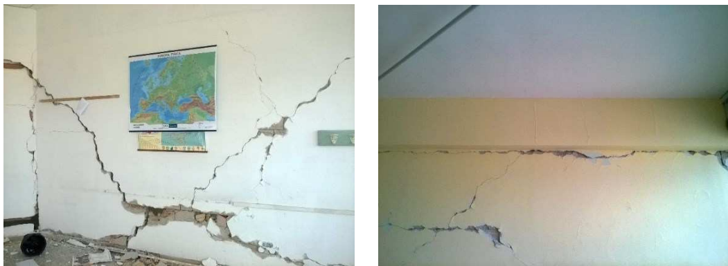
Figure 8.16. Damage to partition walls
