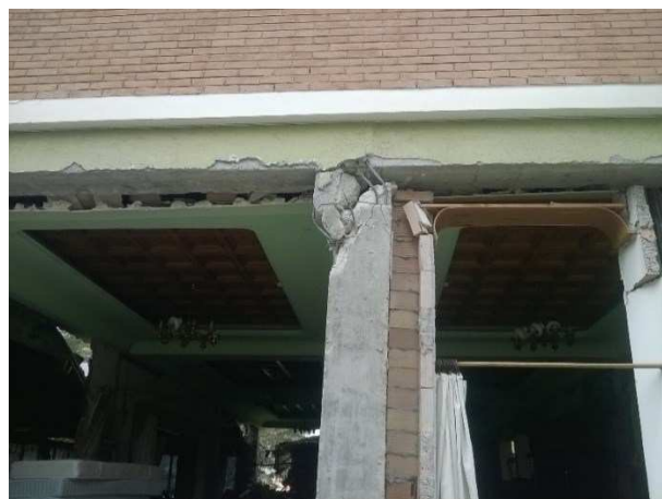
Figure 1.3. Rupture due to weak column-beam joint effect (Amatrice, 2016 Centre Italy earthquake)
