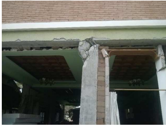
Figure 8.7. Damage to the beam-column joint in the municipality of Amatrice
