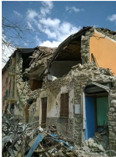
Figure 1.2. Collapse of masonry walls made of poor materials (Grisciano (AP), 2016 Centre Italy earthquake)
