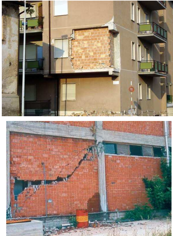
Figure 1.19. Out of plane (left) and in-plane failure (right) of masonry infills
