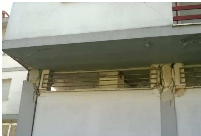
Figure 1.5. Rupture of short columns (Visso, 2016 Centre Italy earthquake)
