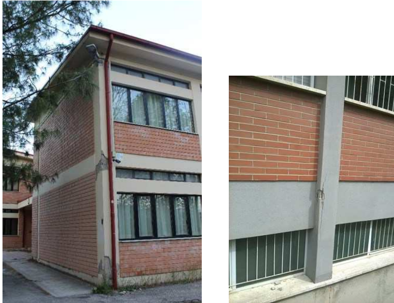
Figure 8.13. Damage to beam-column joints
