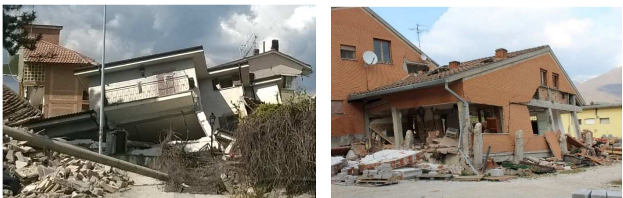
Figure 8.6. Total collapse of buildings due to soft-storey mechanism in the municipalities of Amatrice (left) and Norcia (right)
