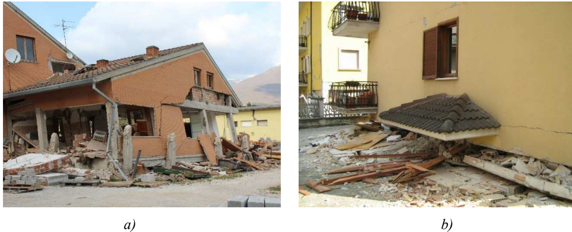
Figure 1.4. Collapse due to soft storey: (a) Norcia, 2016 Centre Italy earthquake; (b) L'Aquila, 2009 L'Aquila earthquake.
