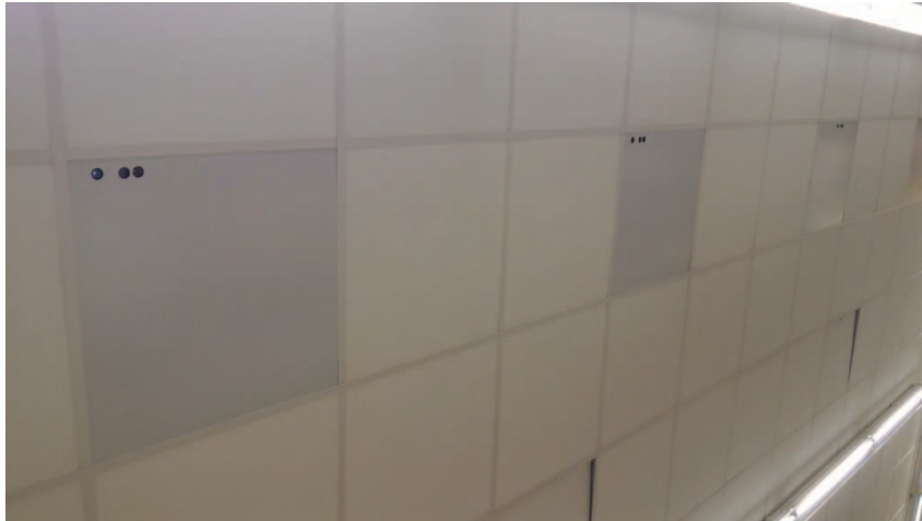
Figure 4.5: An example of RGB-D camera installation on ceiling.
