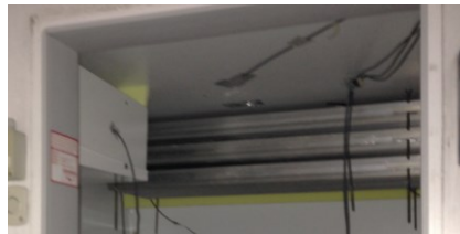
Figure 25: Positioning of the air heat exchanger in the cold room
