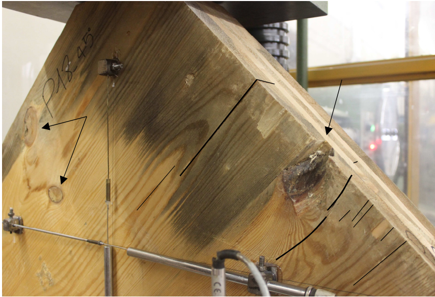
Figure 5.6: specimen S-18 has the shrinkage cracks (black lines) which interest the cross section of the external board and presents knots in the external board (black arrows).
