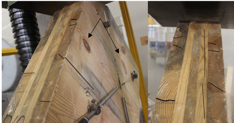
Figure 5.3: specimen S-10 has the shrinkage cracks (black lines) and presents knots in the external board (black arrows).
