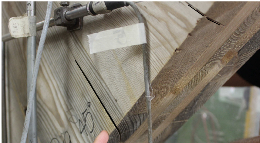
Figure 5.7: specimen S-19 has the shrinkage cracks (black lines) which interest the cross section of the external board.
