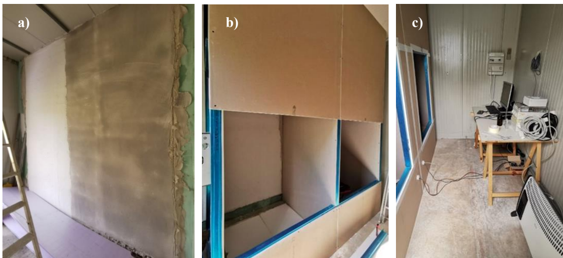
Figure 144. The pilot scale room: a) during the construction phase with the two different finishes applied on the wall (L on the left and U on the right), b) the two testing boxes, and c) the service area with the monitoring data acquisition system.
