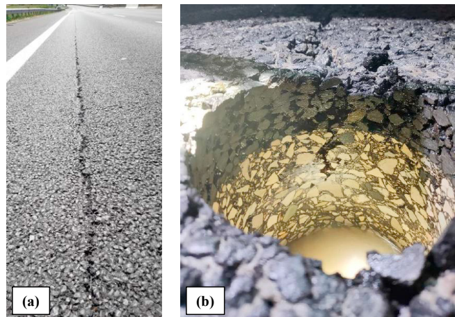
Fig. 1. Typical top-down crack: (a) longitudinal view, (b) transverse view.
