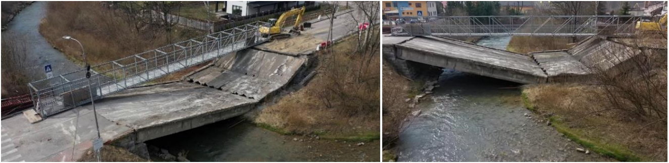
Figure 2: Collapsed bridge in Trstena, Slovakia (2020) (Pallo, 2020)
