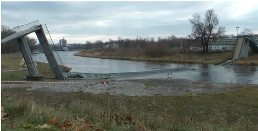
Figure 1: Collapsed footbridge in Prague, Czechia (2017) (WEBVIZE.cz, 2017)
