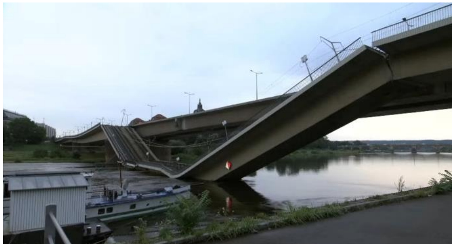
Figure 3: Collapsed bridge in Dresden, Germany (2024) (Iamcivilengineer, 2024)
