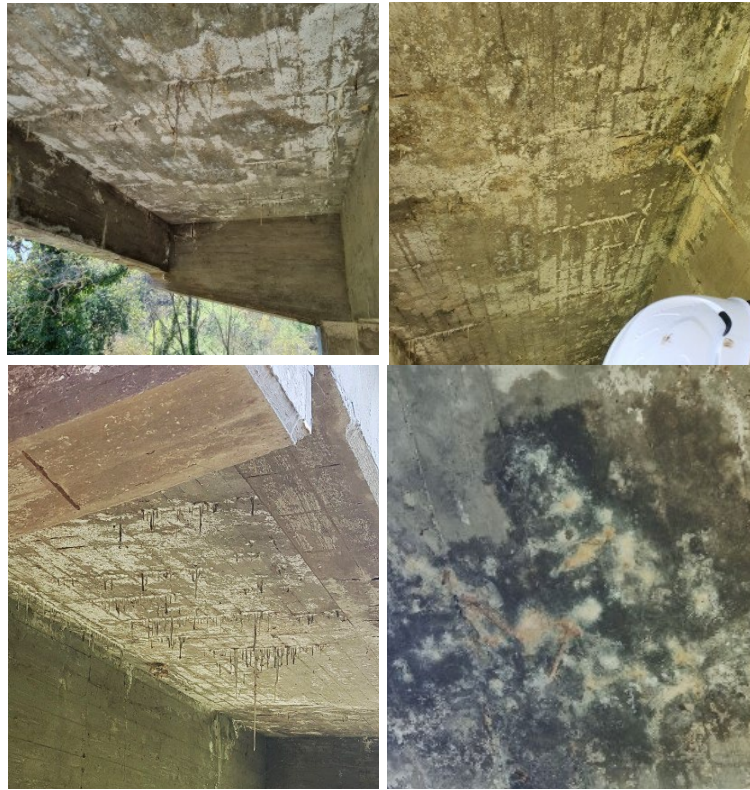
Figure 34. Efflorescences and stalactites on concrete slabs.
