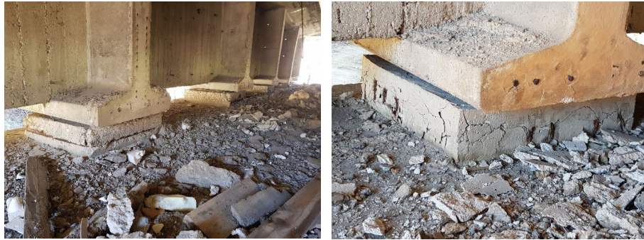
Figure 38. Cracks and concrete degradation on the support pedestals.
