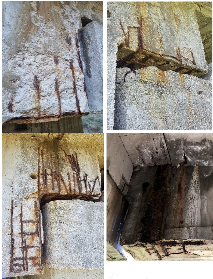
Figure 49. Damages on dapped-end beams due to water infiltration.
