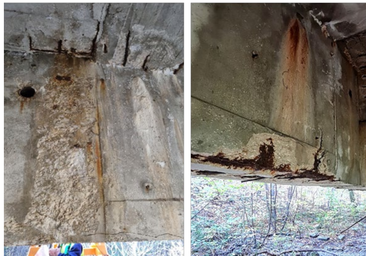
Figure 48. Damages on RC beams due to water infiltration: calthemite flowstone, reinforcement corrosion and concrete spalling.
