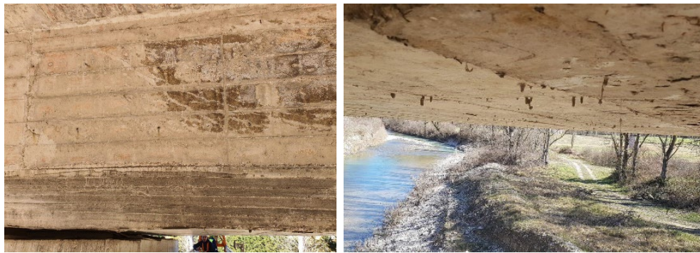
Figure 51. Crack along the prestressed cable paths in the beam ends (left) and water stagnations inside the box girder (right).
