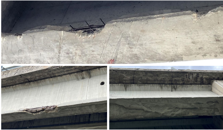
Figure 42. Impact damages on the bottom flanges of the beams and crack patterns on concrete.
