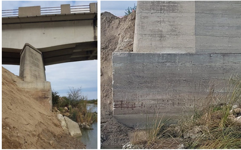
Figure 45. Central pier scour (left) and diagonal cracks on the pier foundation (right).
