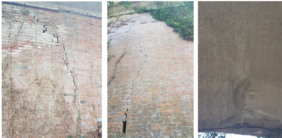
Figure 18. Cracks along the masonry texture on abutments and concrete arch.
