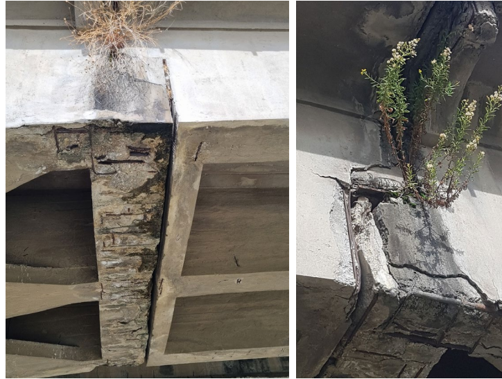
Figure 44. Concrete degradation, cover spalling and steel corrosion on dapped-beam ends.
