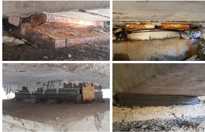
Figure 39. Oxidation and corrosion of metal support devices and crushing phenomena on reinforced rubber bearings.
