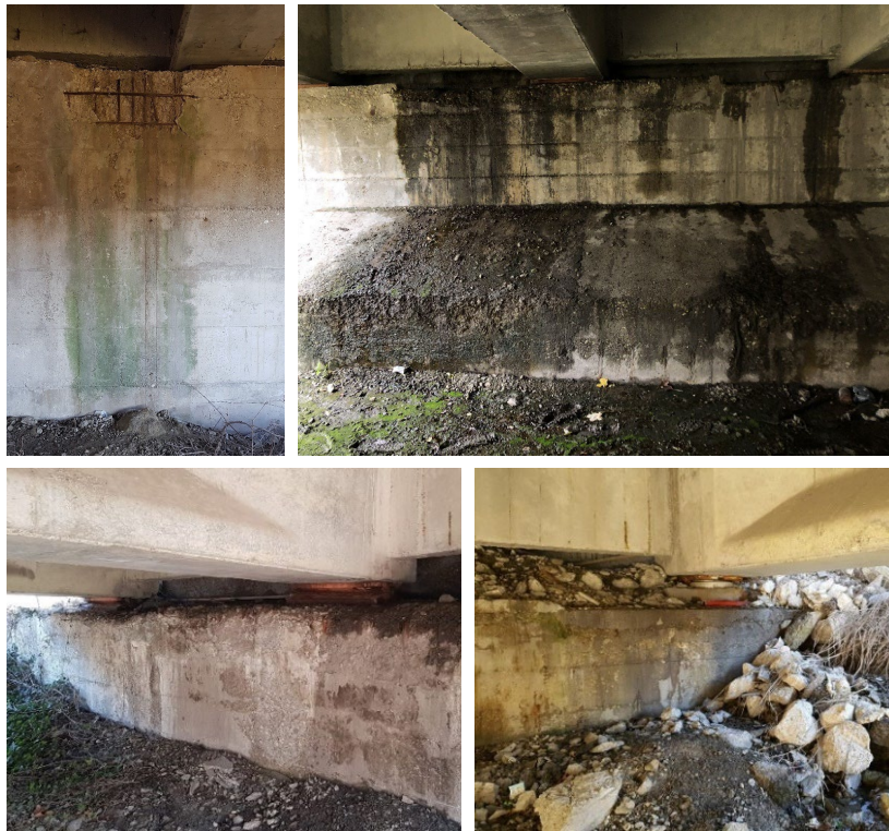
Figure 40. Photos of abutments affected by water infiltration from road embankment and pavement.
