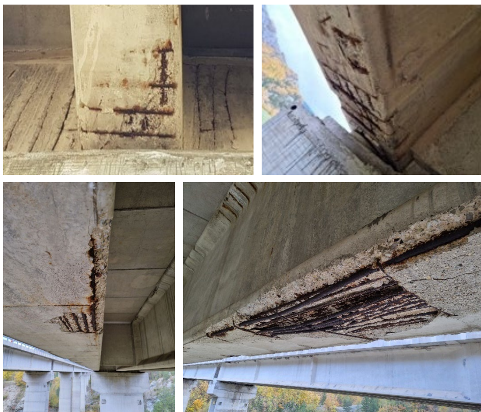
Figure 41. Concrete spalling and steel corrosion on Prestressed RC beams.
