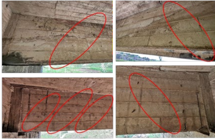
Figure 28. Diagonal cracks on the support zones of the RC beams.
