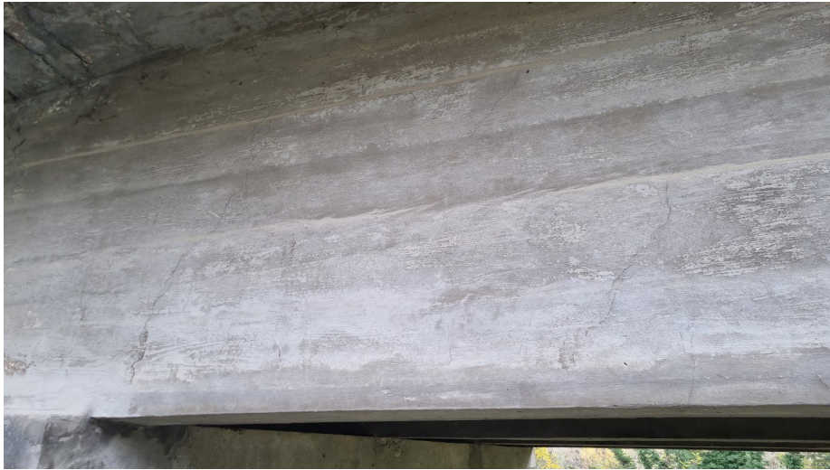
Figure 33. Bending cracks of the external concrete beam near to the support.
