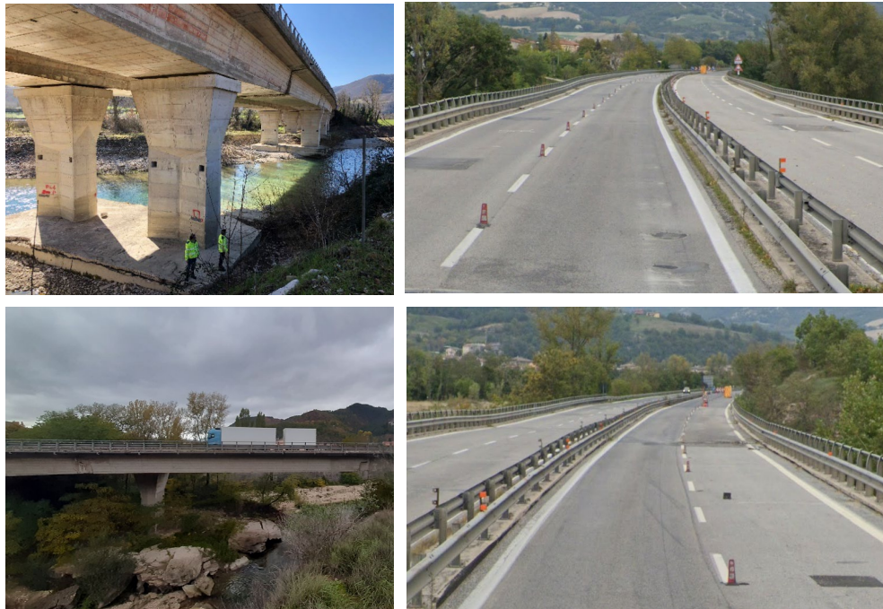
Figure 52. Permanent deflection of the suspended spans.
