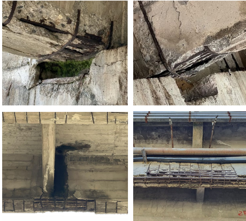
Figure 26. Corrosion and stirrup failure on the support section (upper) and on mid-span section (lower)
