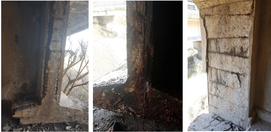
Figure 43. Concrete spalling and corrosion on the beam ends.
