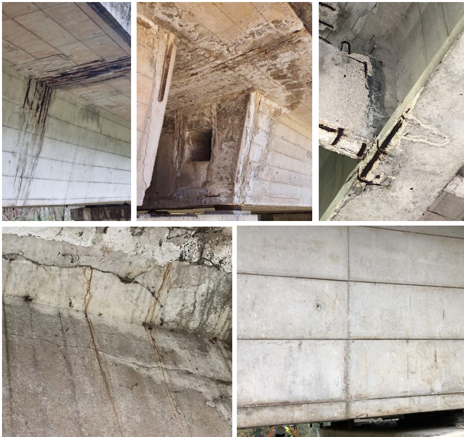
Figure 47. Humidity traces, concrete degradation and steel corrosion on box girders (upper) and cracks along the post-tensioning cable paths (lower).
