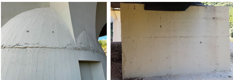
Figure 22. Concrete honeycombs on pier (left) and shrinkage cracks on concrete cap (right),
