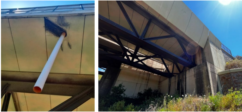
Figure 20. Water infiltrations on the concrete slab (left) and on the abutment (right).
