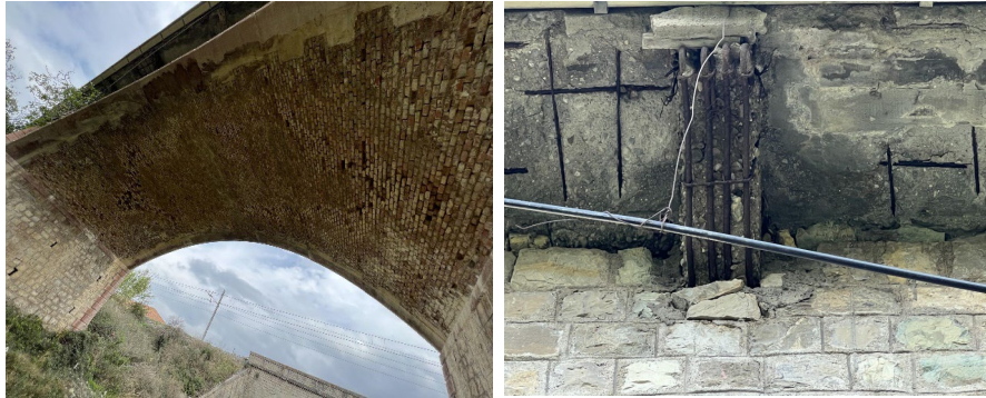
Figure 16. Material degradation on the arch (left) and cover spalling and reinforcement corrosion on the concrete slab (right).
