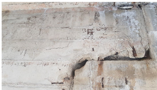
Figure 103. Cracks on the dapped-end beam.
