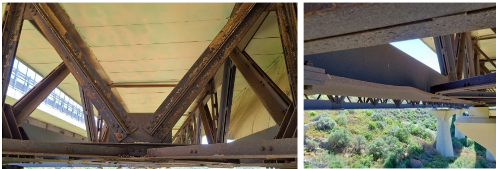
Figure 21. Steel corrosion of the Corten steel (left) and impact damages on beams (right).
