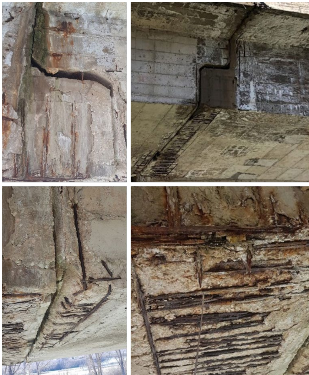
Figure 53. Damages on box dapped-end beams due to water infiltration.
