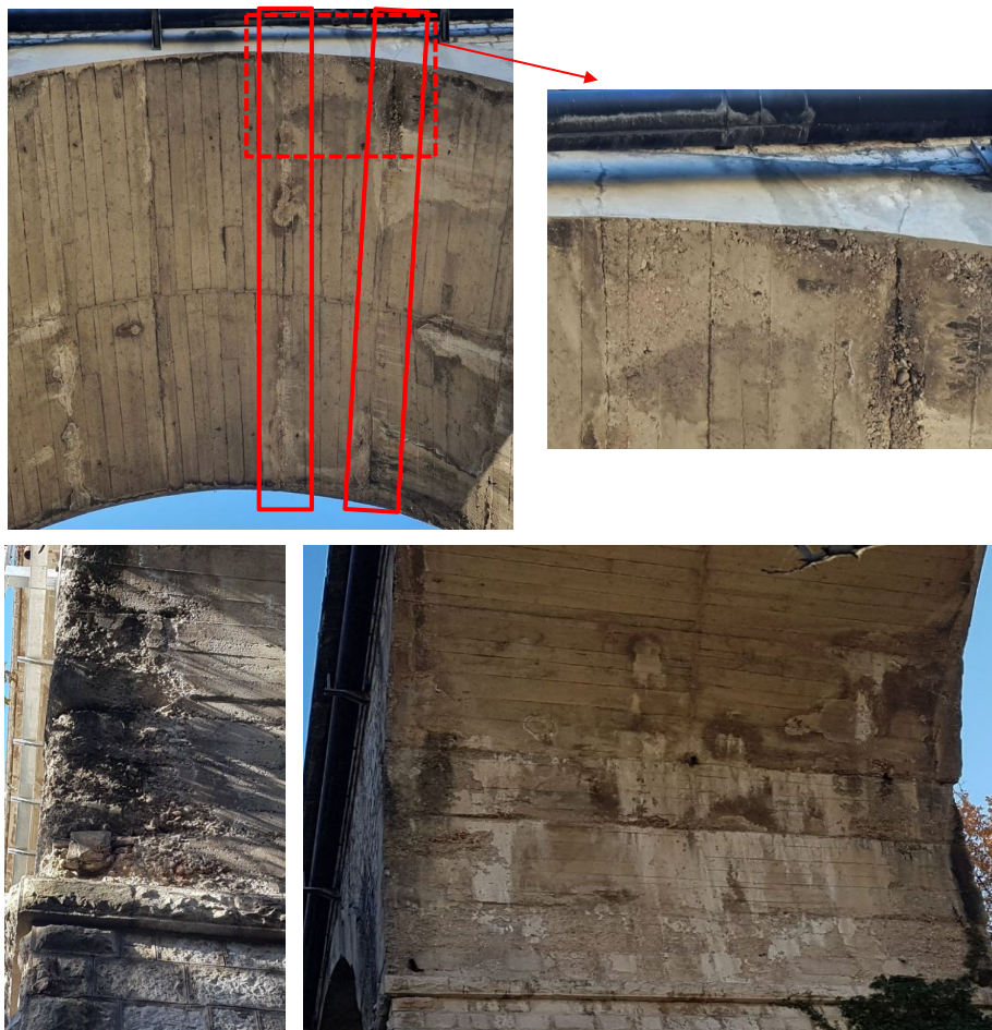
Figure 30. Transversal cracks on concrete arches (upper) and concrete degradation and humidity (lower).
