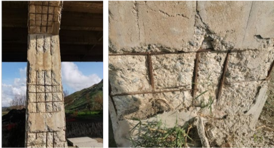
Figure 27. Concrete cover detachment and stirrup failures on concrete pier.
