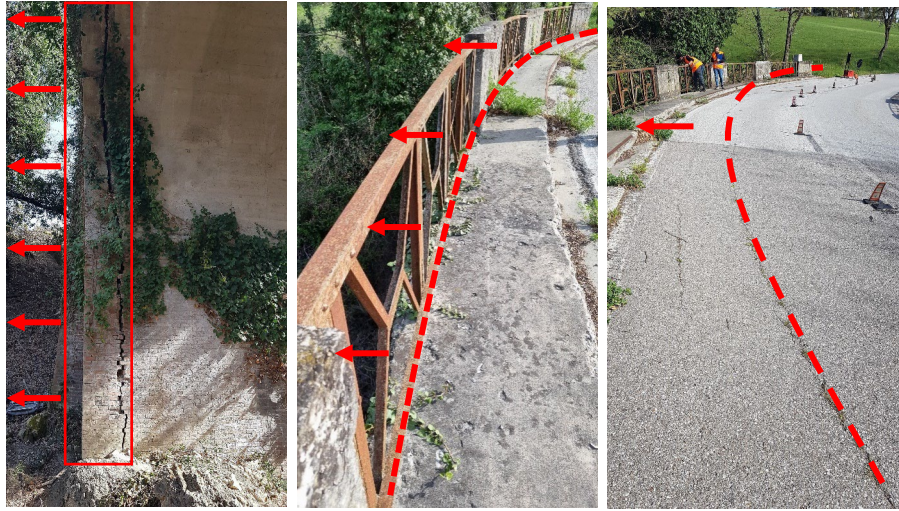
Figure 17. Out of plane failure mechanism of the curved masonry arch bridge.
