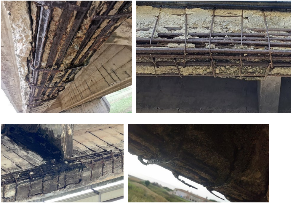
Figure 25. Reinforcement corrosion and stirrups failure in the mid-span section of RC beam.
