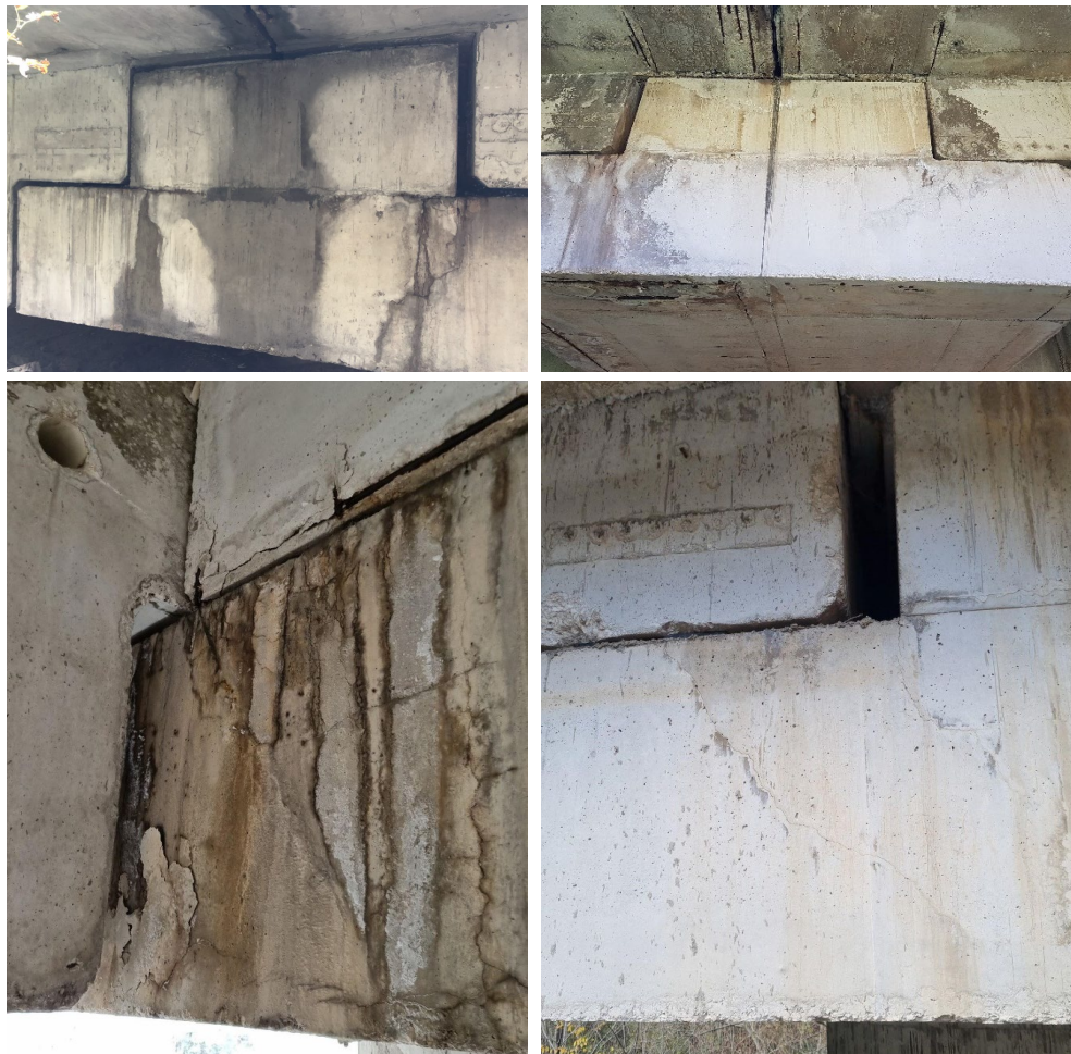
Figure 50. Diagonal cracks on the dapped end of the pier caps.
