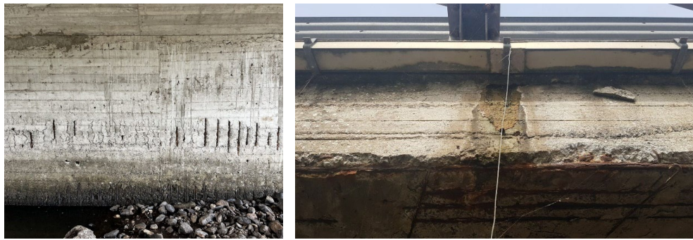
Figure 24. Covert spalling and reinforcement corrosion.
