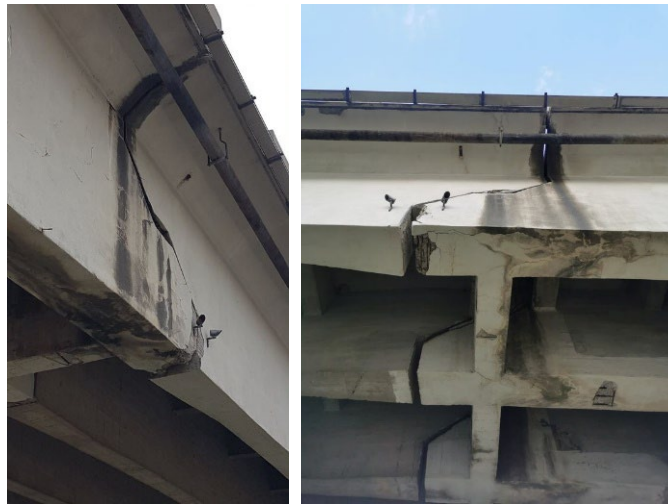
Figure 46. Compression cracks and water traces on the dapped-beam ends.
