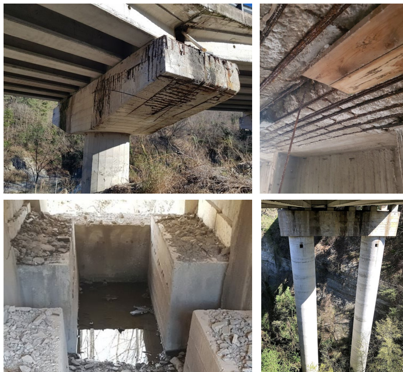
Figure 37. Concrete spalling and reinforcement corrosion on pier caps and water infiltrations and stagnations on the top of the cap.
