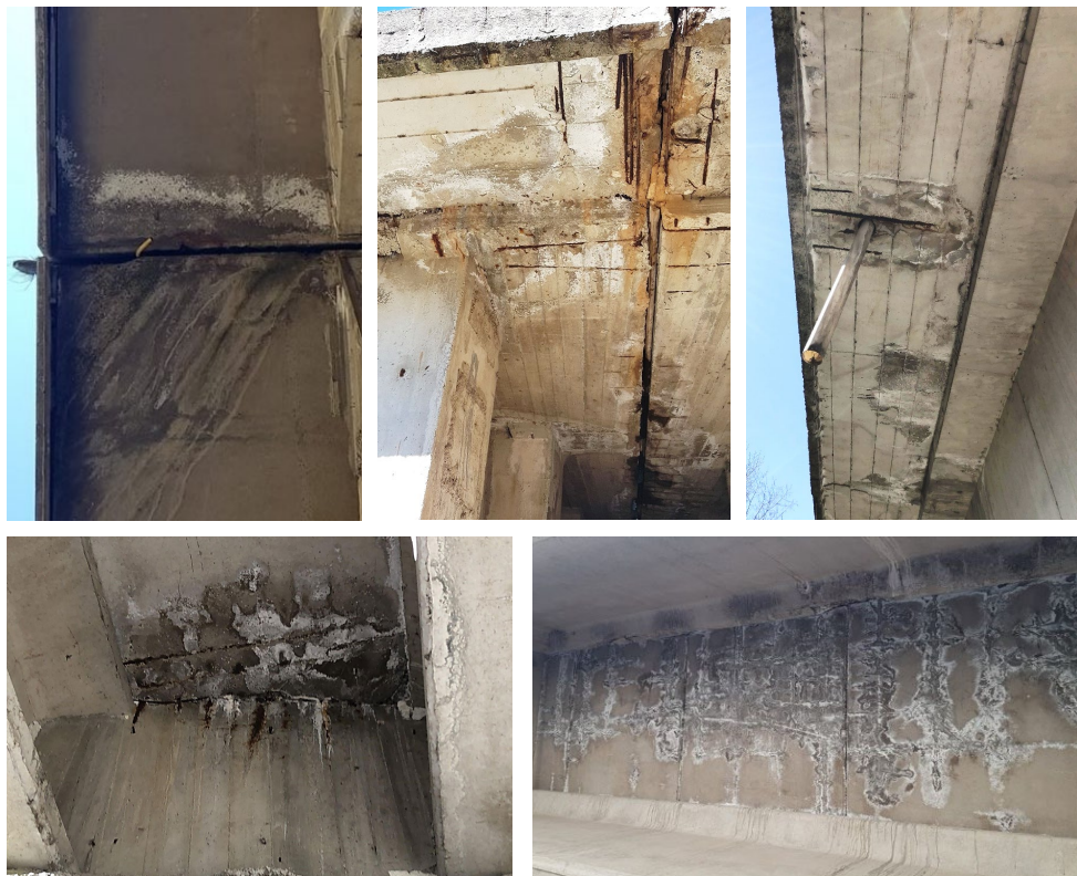
Figure 36. Photos of moisture, concrete spalling and steel corrosion in the concrete slabs.
