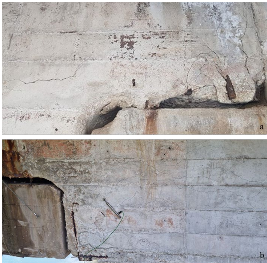
Figure 55. Potential failure mechanism of the box dapped-end beams.
