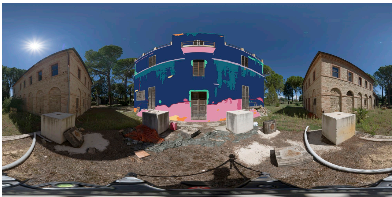
Figure 3. The Villa Leonardi spherical panorama. View of the rear façade displaying the decay information according to ICOMOS-ISCs glossary.
