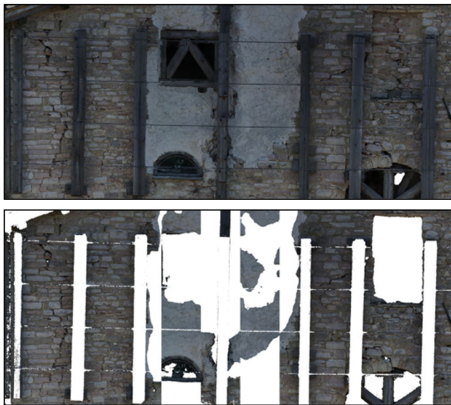
Fig. 13. Upper part of the north façade (visible bands, top), and the same after the application of the depth-based filter (bottom).
