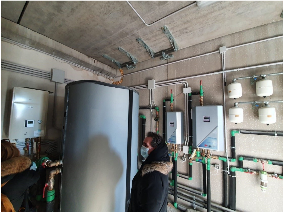
Figure 60: General overview of the central heating plant
