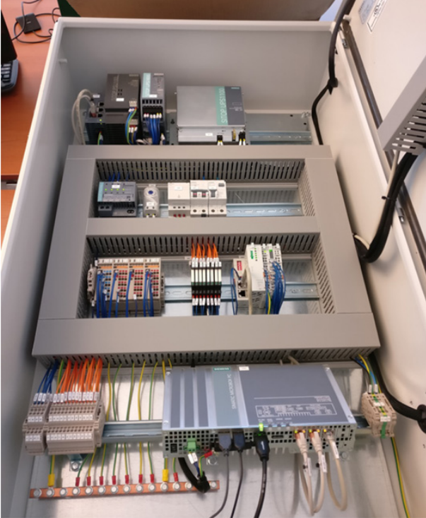
Fig. 2. Real control unit cabinet.
