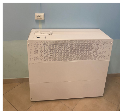
Figure 5. HRV unit installed in the monitored classroom (Innova HRC+ 60 H/HV).
