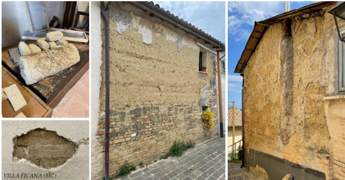
Figure 73: Examples of the three earthen masonry typologies considered: the Cob at the top left, the Adobe at the bottom left, and the Ramed earth in the two buildings on the right. Photos taken at the Ecomuseum of Villa Ficana (MC).
