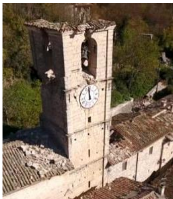
Figure 2. Belltower in Castelsantagelo, damaged by the earthquake in 2016 (confined tower)
