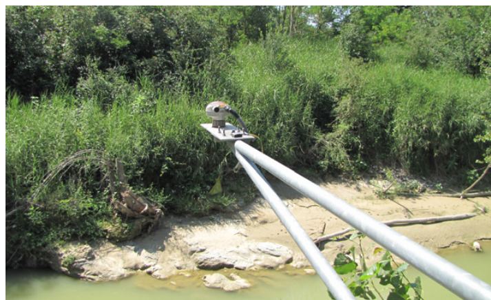
Figure 7. Example of a gauge ultrasonic sensor used to acquire the stages measurements (SITRANS Probe LU, Table 1).
