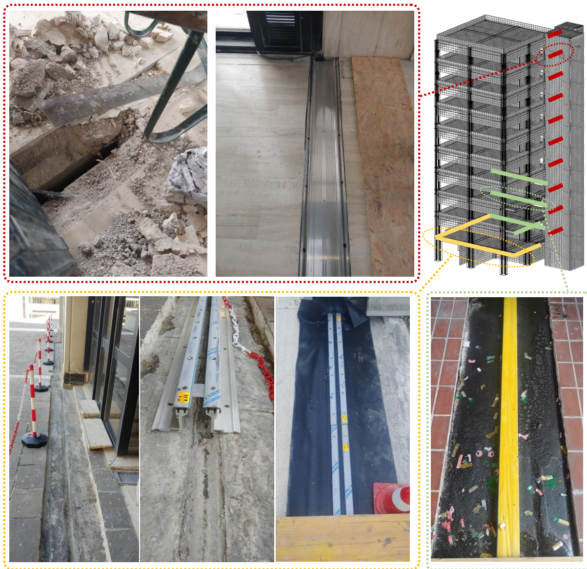
Figure 7-20: Some photos of the retrofit works carried out on the tower structural joints.
