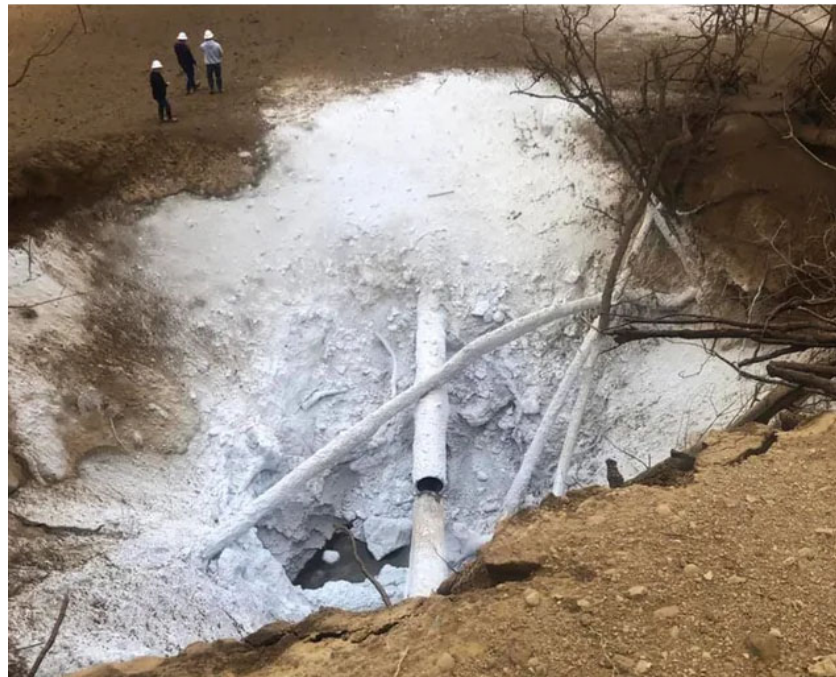
Figure 1. CO 2 pipeline rupture and dry-ice formation occurred in Yazoo County in 2020 (Mississippi Emergency Management Agency—MEMA) [22].
