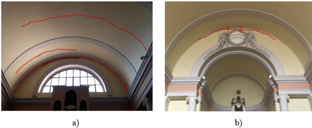
Figure 6.8: Camorcanna vault damage survey: in the middle and with the facade (a) and with the wall delimiting the apse (b)
