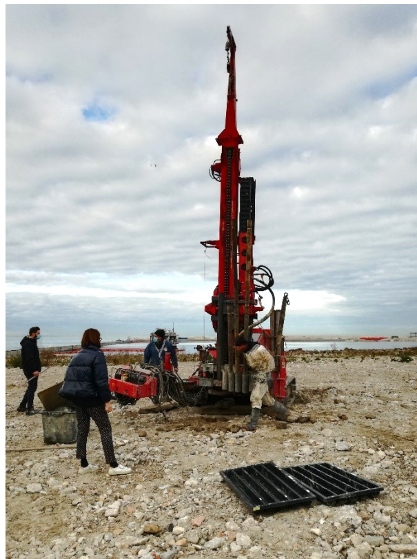
Figure 6.22. The drilling rig S30 (by Mori s.r.l.), mounted on a crawler truck, during the geotechnical campaign after the embankment removal.
