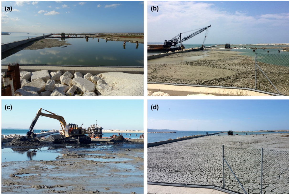
Figure 4.12. Filling of the test field sector: (a) start-up phase; (b) filling operations from the sea-side of the CDF; (c) spreading of the disposed sediments; (d) surficial crust formed after water evaporation.
