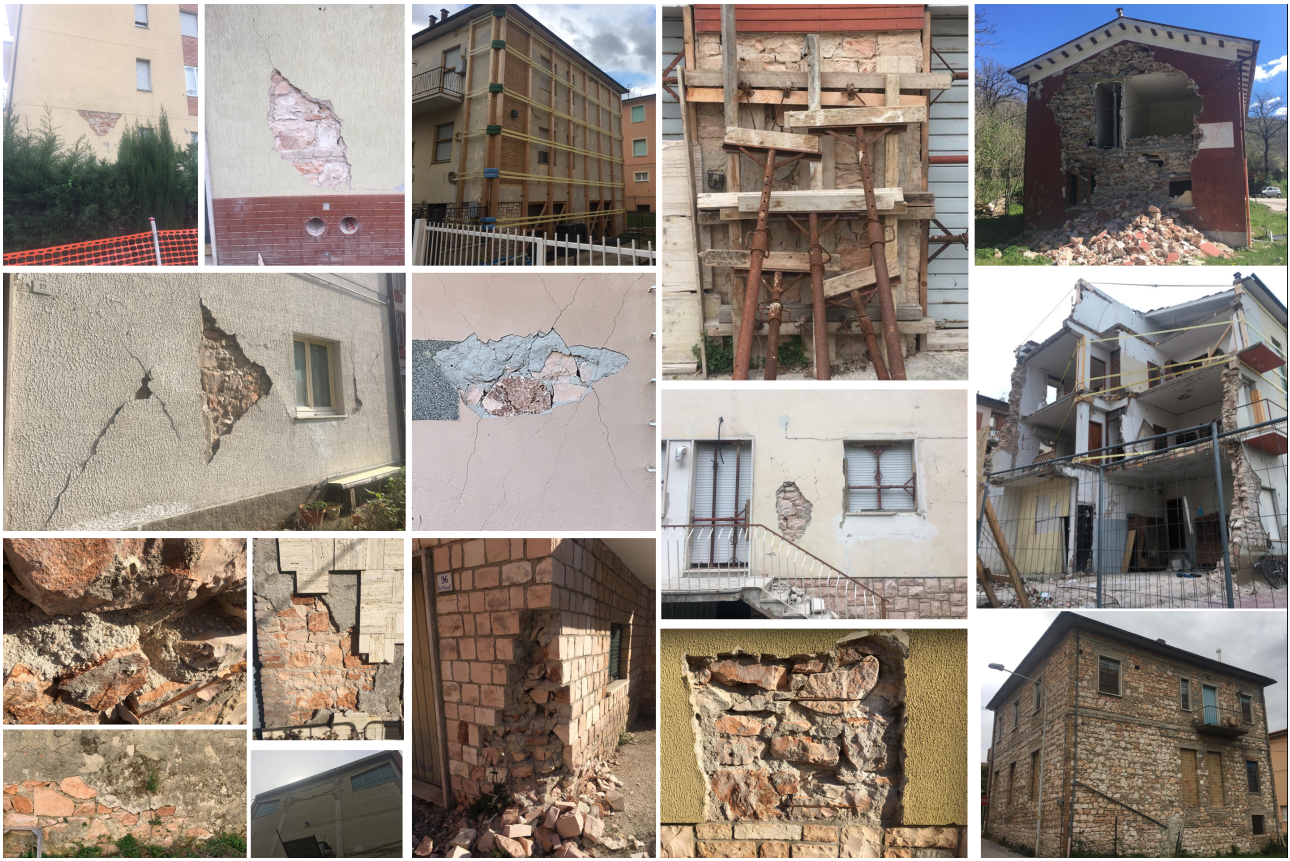
Figure 1 - Damage on “Scaglia Rossa” masonry structures after Central Italy seismic sequence.
