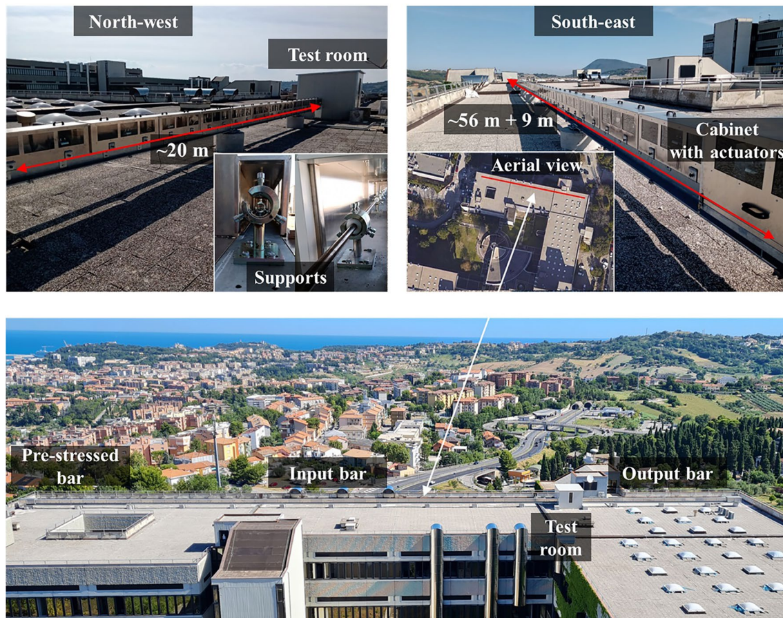
Fig. 8 Facility installed on the roof of Engineering Building at Marche Polytechnic University (Lat.43.58776°N, Long.13.51667°E)
