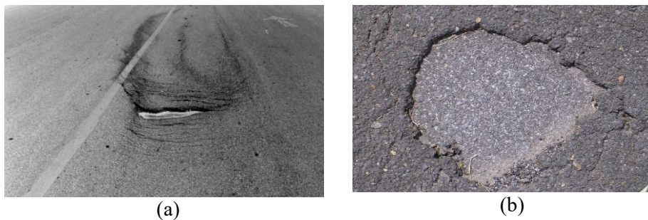
Figure 2.3. Premature failures: a) Slippage; b) Delamination.
