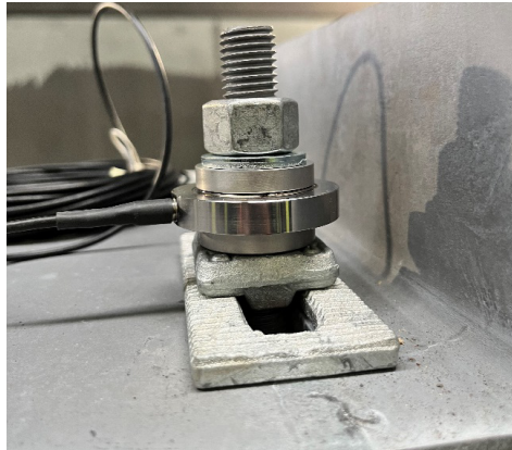
Figure 13. Zoom on the force washer installed on the bracket's bolt.
