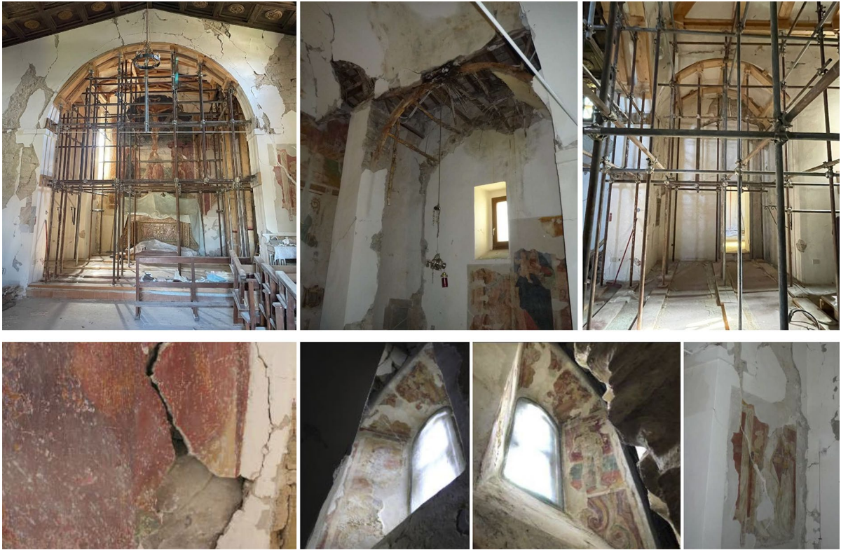
Fig. 3 Detail of the damage inside the church and of the windows near the bell tower placed at 5 cm from the back wall
