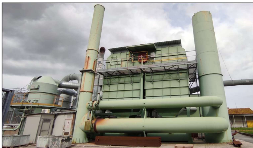
Fig. 6 Regenerative Thermal Oxidizer and wet scrubber
