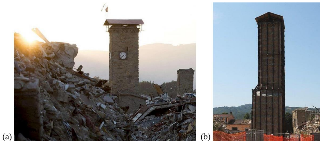
Figure 36 – View of the tower after the first securing operation (a) and after the interventions carried out after the first securing operations (b).
