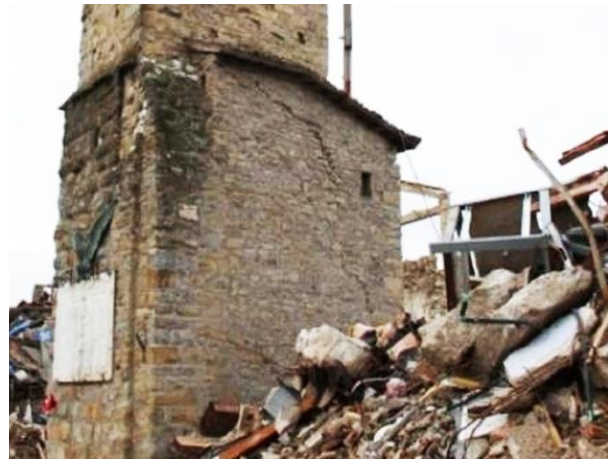
Figure 35 – Details of the crack pattern developed on the annex of the tower after the seismic sequence in 2016.
