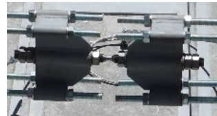
(e) Close-up of the fuse bar
