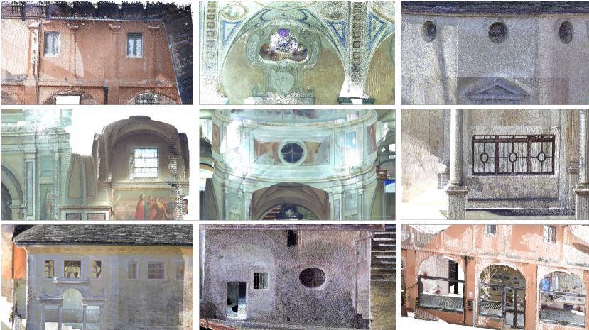
Figure 4.6: Different typologies of windows and doors. For the latter, their opening has sometimes affected the points acquisition.
