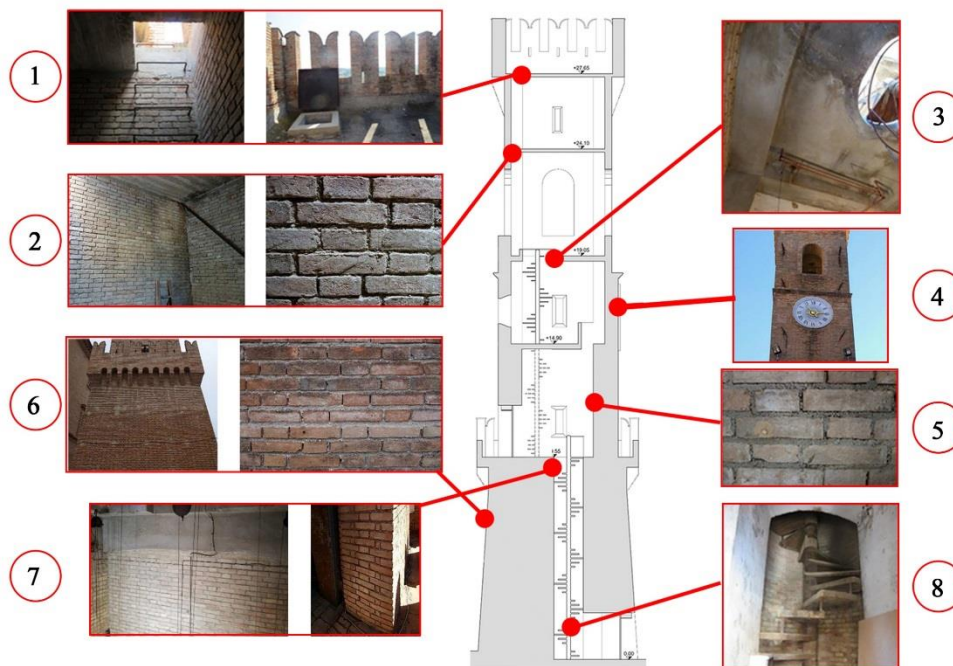
Figure 12: Excerpts from the photographic survey of the tower: (1) Trapdoor accessing the upper level and connecting iron ladder; (2) close-up of the 4th level brickwork; (3) concrete slab of the 3rd floor with ladder opening; (4) particular of the reinforcement intervention with tie rods; (5) close-up of the 2 nd level internal brickwork; (6) external brickwork of the 1 st level; (7) basement brickwork; (8) spiral staircase at the entrance level.
