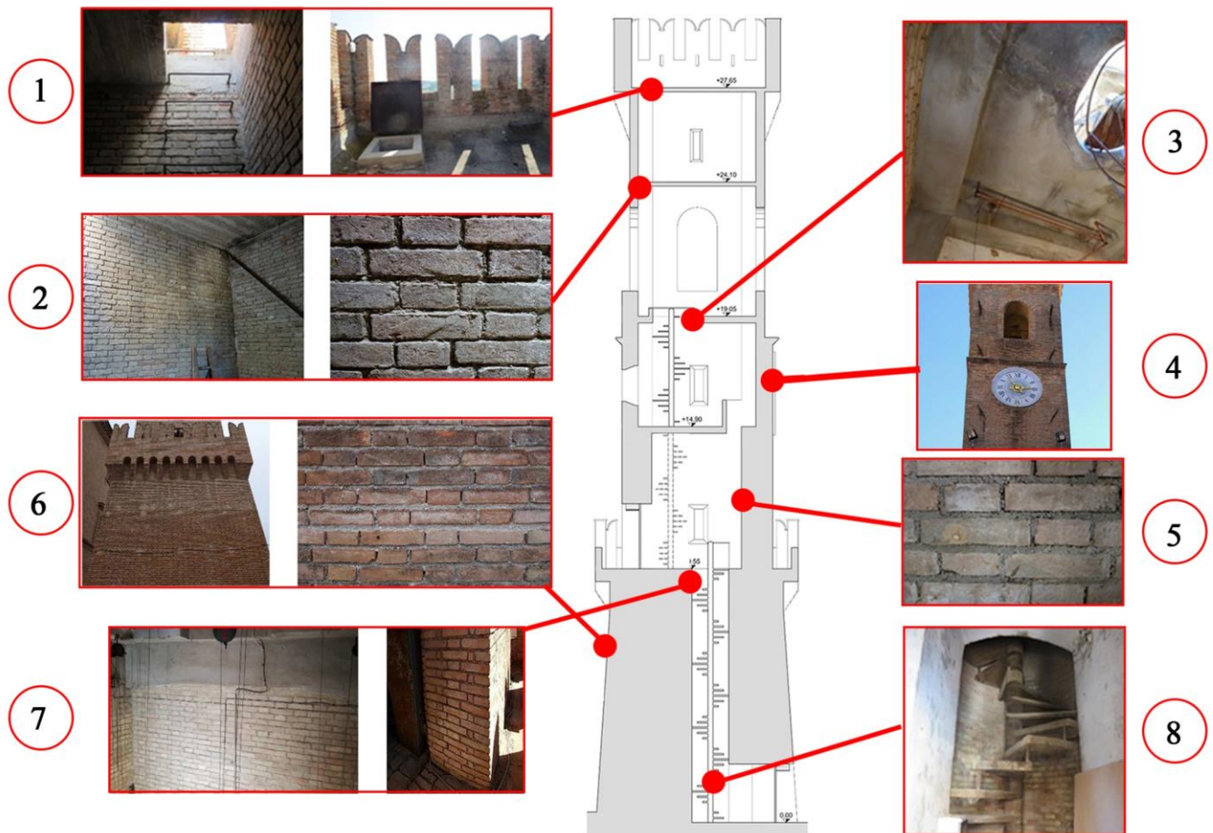
Figure 4 – Excerpts from the photographic survey of the tower:(1) trapdoor accessing the upper level and connecting iron ladder; (2) close-up of the 4 th level brickwork; (3) concrete slab of the 3 rd floor with ladder opening;(4) particular of the reinforcement intervention with tie rods; (5) close-up of the 2 nd level internal brickwork; (6) external brickwork of the 1 st level; (7) basement brickwork; (8) spiral staircase at the entrance level.
