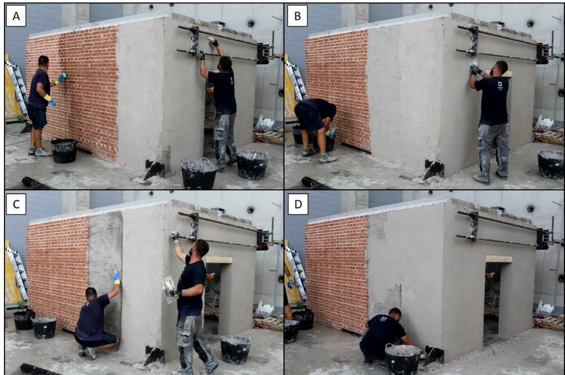
Figure 4.2 Construction phases of TRM application. a) Cleaning of the masonry support; b) Application of the first layer of mortar; c) Positioning of the glass textile and finally; d) Application of the second layer of mortar.
