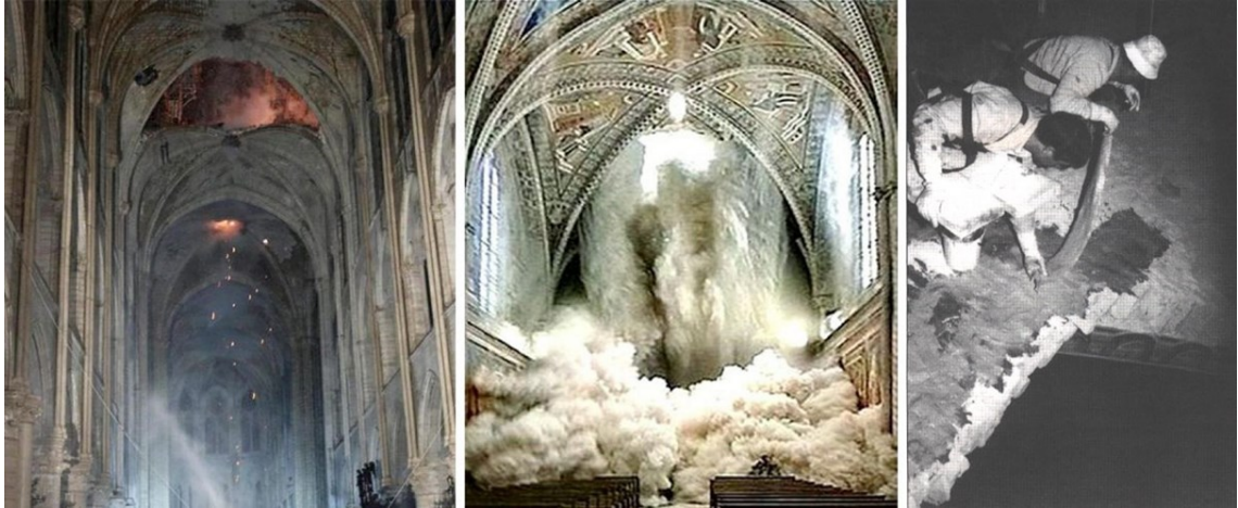
Figure 2.11 Collapse and reinforcement of Gothic vaults of San Francesco Church in Assisi
