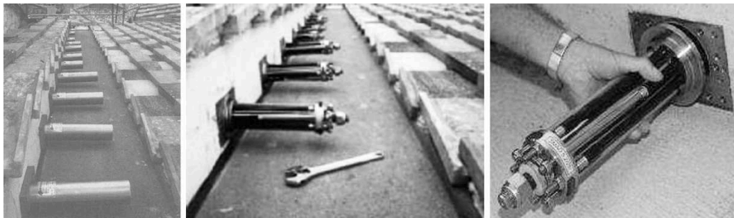
Figure 2.3 - Shape memory alloy devices installed in the Basilica of San Francesco, Assisi (Castellano, 2005)
