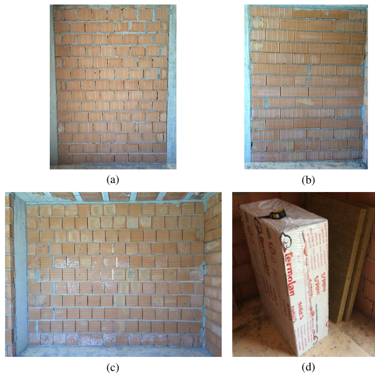
Figure 2.6 Infill masonry walls typology: (a) wall W1-A, (b) wall W2-A, (c) wall W3-A, (d) glass wool used inside the wall W2-A.
