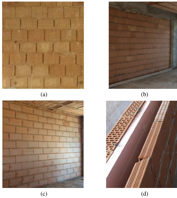
Figure 2.2 Infill masonry walls typology: (a) wall W1-F, (b) wall W3-F, (c) wall W2-F, (d) section of the wall W2-F.
