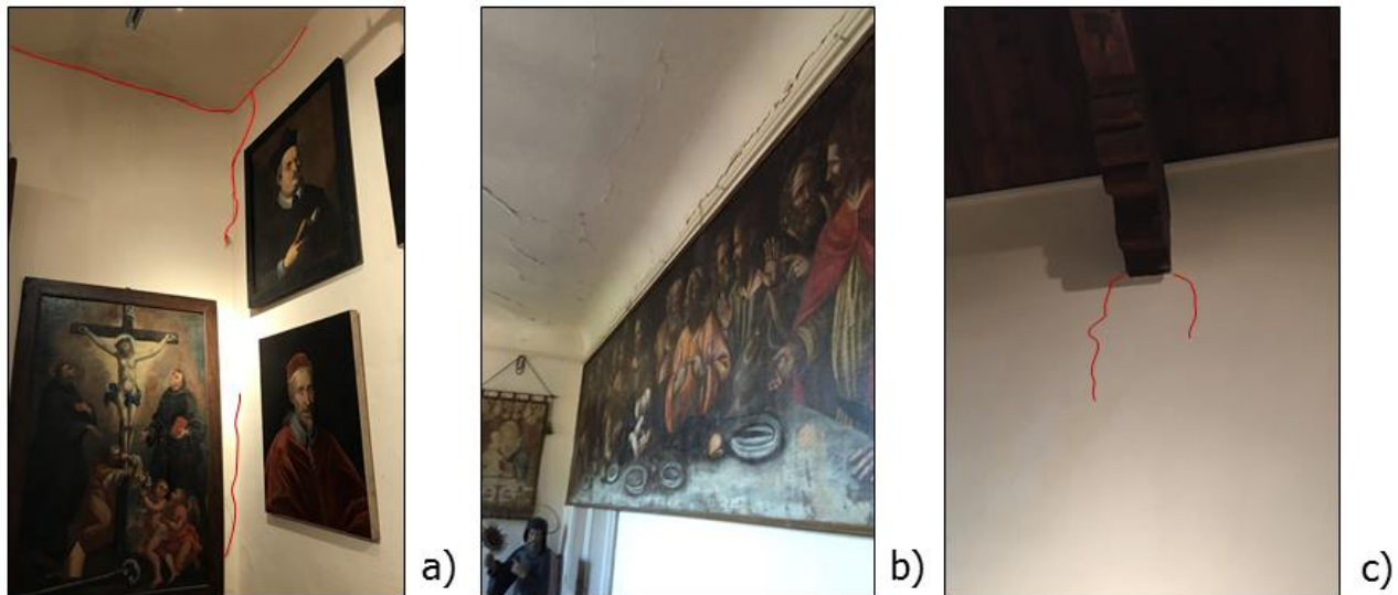
Figure 4. Some damages in the camorcanna and in the connection between transversal walls (a), only in the camorcanna (b) and in the connection between wooden beams and walls of the facades (c).
