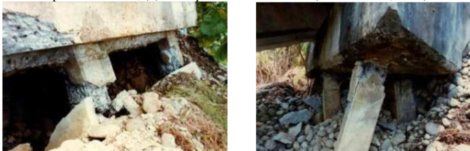
Figure 1-3 (a) Preferential damage to front batter piles of Rio Banano bridge; (b) failure of Rio Viscaya Bridge Piles, during the 1991 Costa Rica earthquake (after Priestley et al., 1991)
