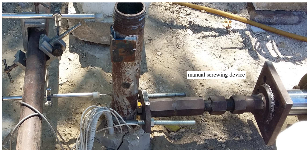
Figure 4-32 Details of the coupling between screwing device and reaction pile during test on P1
