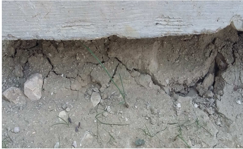
Figure 5-40 Superficial soil cracks around the pile
