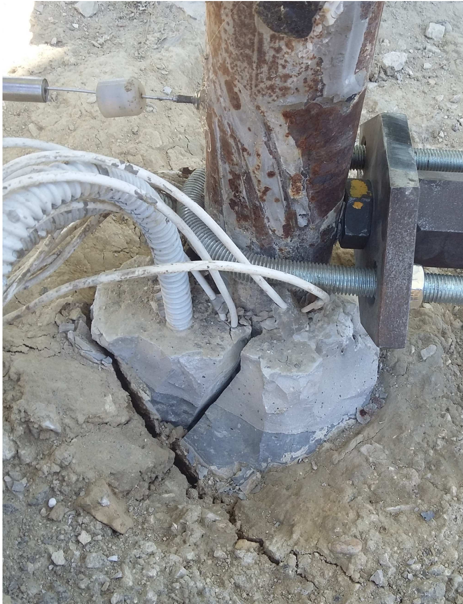
Figure 5-19 Gap at the end of the first loading cycle on P1
